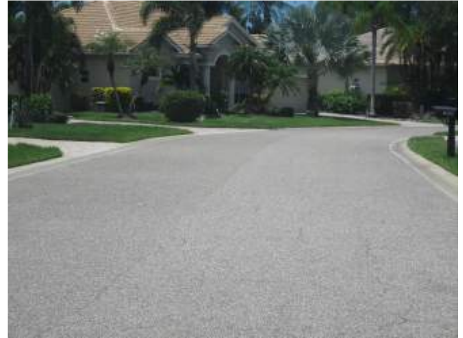
Southwest side of Camden Harbour viewing north, minor cracks
