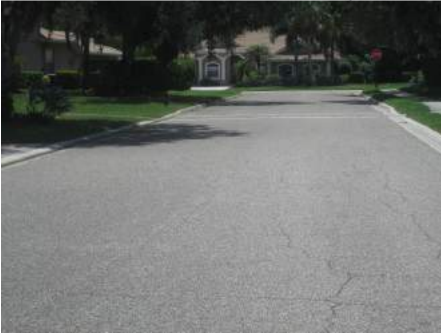
West side of Camden Harbour viewing south, minor longitudinal cracks
