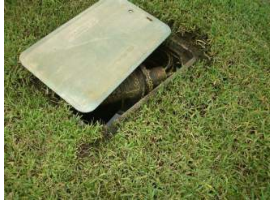
Phone box next to condo's full of water with top displaced
