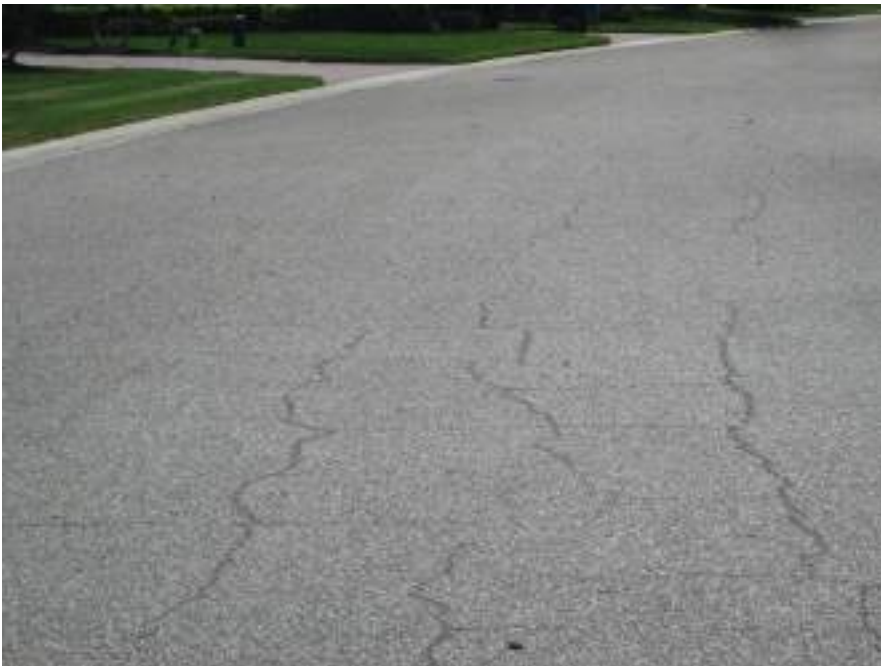
North side of Camden Harbour viewing east, minor longitudinal cracks
