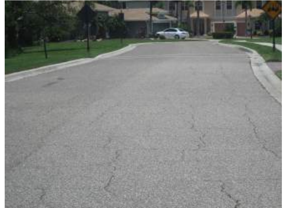
West side of Camden Harbour viewing north, minor longitudinal cracks
