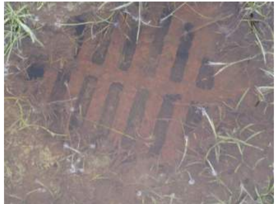
Drain Inlet southwest of sand trap
