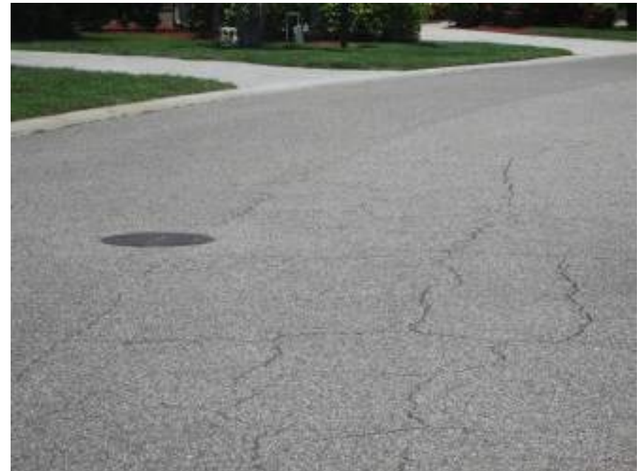
Southwest side of Camden Harbour viewing north, longitudinal cracks
