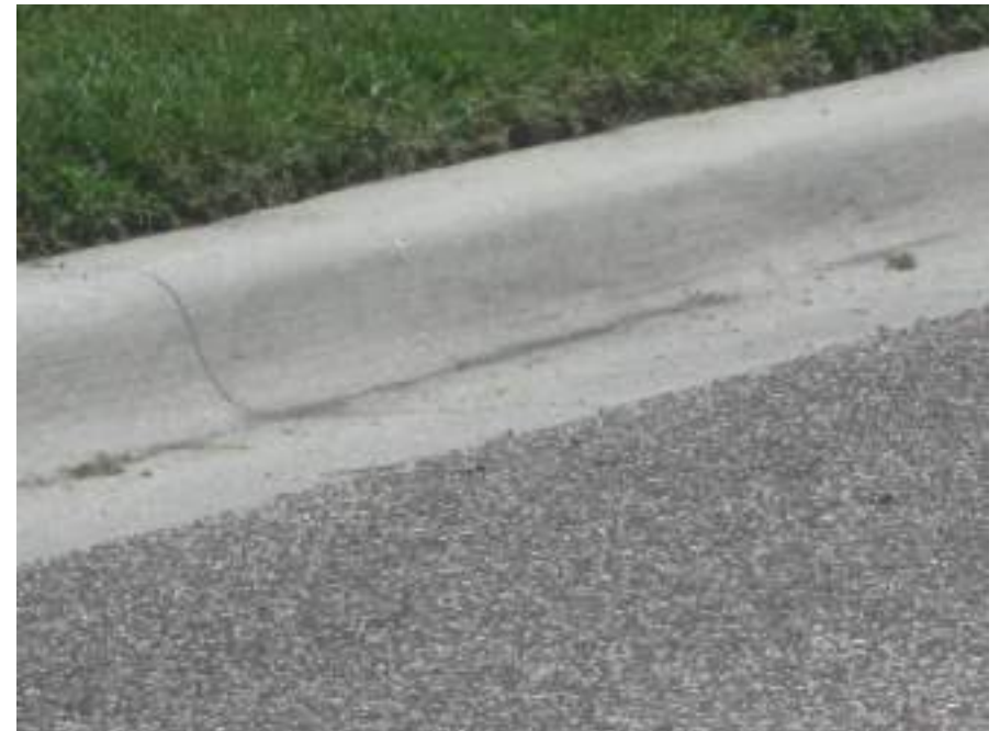
Curb line along west side of Camden Harbour, minor wearing at curb
